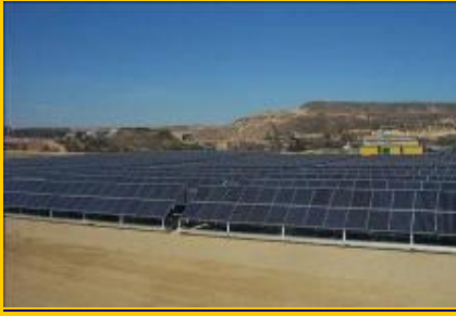
Photovoltaic Installation in Aznalcollar, Sevilla © Andalusian Energy Agency
