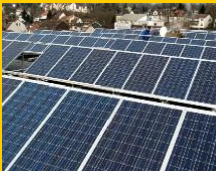
PV plant on the roof of the Tower School in Dudweiler © IZES gGmbH
