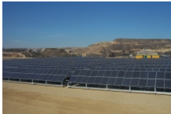
Photovoltaic Installation in Aznalcollar, Sevilla
