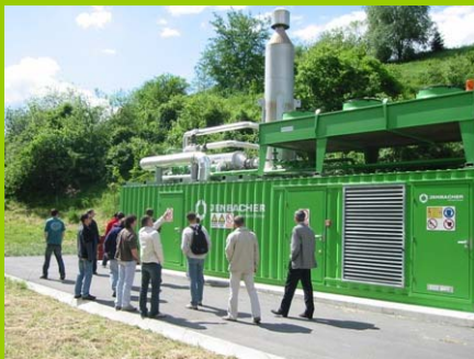
Landfill gas engine for electricity production in the Municipality of Celje
